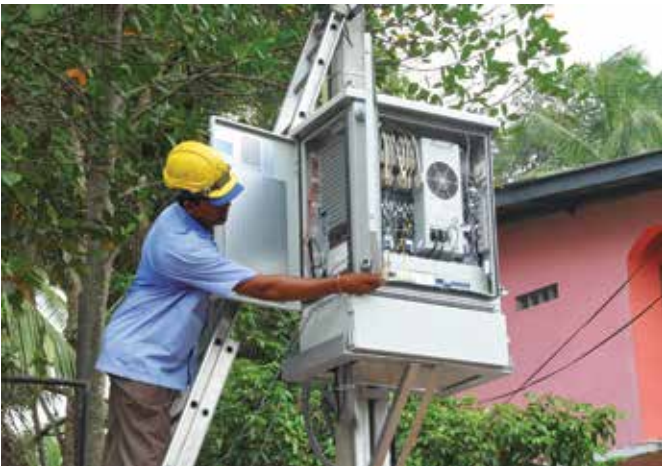
Inspecting MSAN of i-Sri Lanka project
