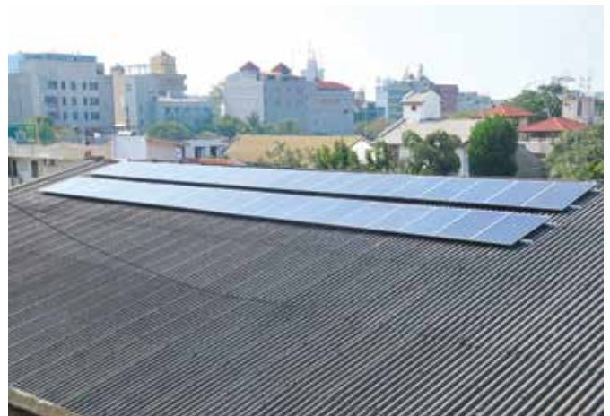
Solar Power Systems in place at SLT premises
